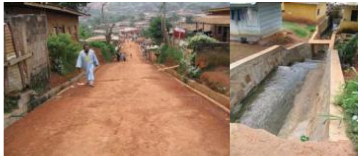
Road levelling and drainage projects, ERA -Cameroun in Yaounde VI (2004) Photo by R. Skinner
